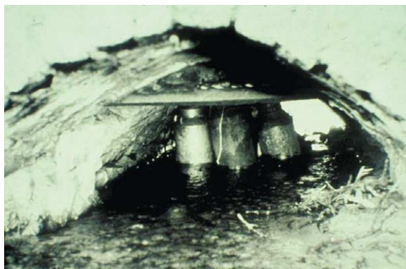
Figure 24 Typical culvert bomb beneath a road. Homemade explosive has been packed into a number of milk churns ready for detonation.
